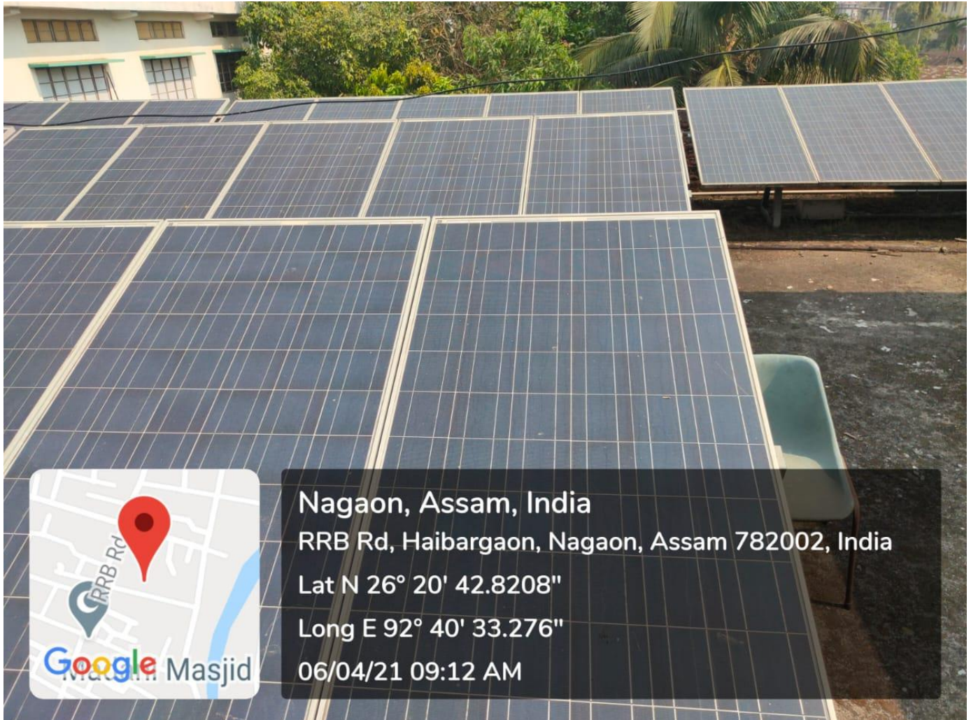
Fig: Grid connected solar PV plant
